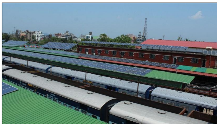
Figure 2: Rooftop solar installations at a railway station, illustrating the integration of distributed renewable energy within public transport infrastructure under India's decarbonisation strategy
