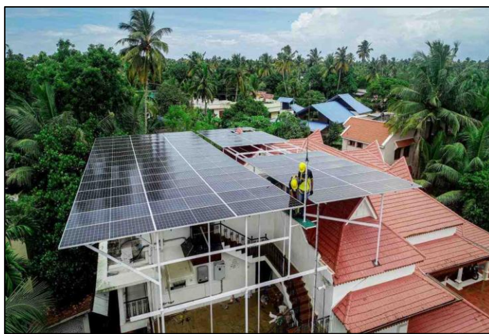
Figure 3: Residential rooftop solar deployment supported by subsidy schemes and green credit mechanisms, reflecting the role of distributed energy in reducing grid dependence and household carbon footprints
